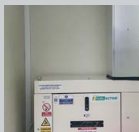
Warm room/ Generator area
