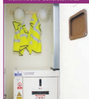
Warm Room / Generator Area
