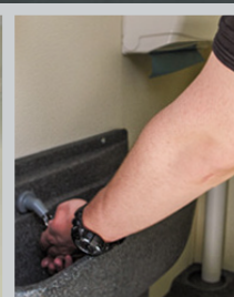
Delivery of hot water
