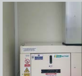
Warm room/ Generator area
